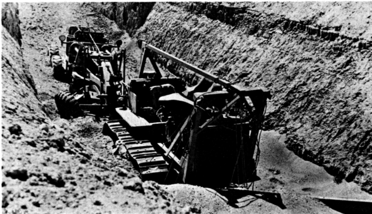
Figure 12.40c. Earth-moving equipment protected in deep trench at right angles to blast wave motion (30 psi overpressure).
